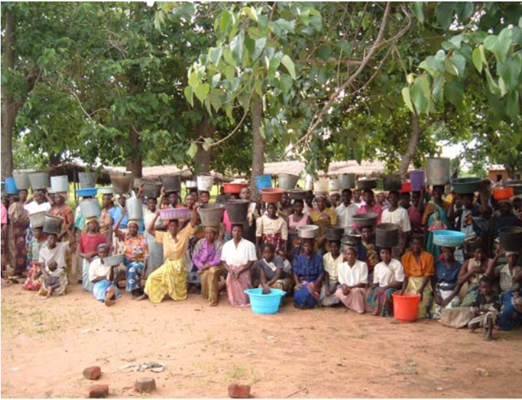
These are women from the village where one of the schools is being built. They are carrying sand and gravel for the foundation of the school.
